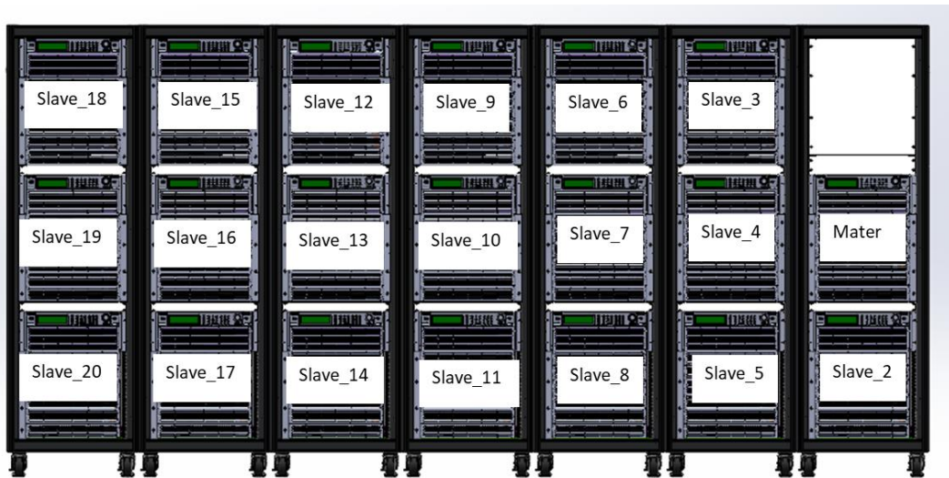
Figure F-9 Setup of 20 Units DC Electronic Load
