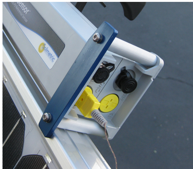
Figure 23. Thermocouple plugged into the TC1 connector.
