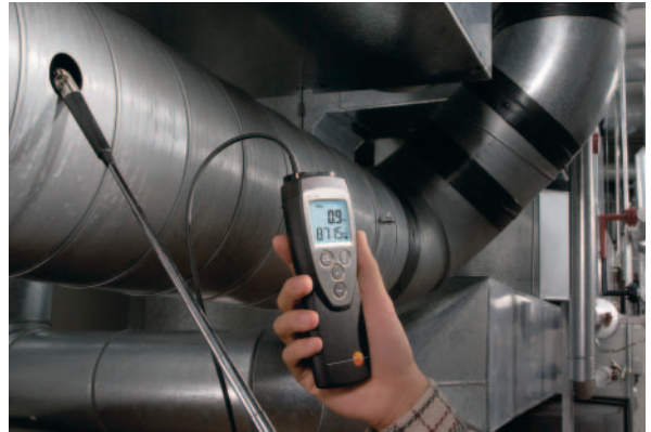
testo 416 monitoring the volume flow of exhaust air
